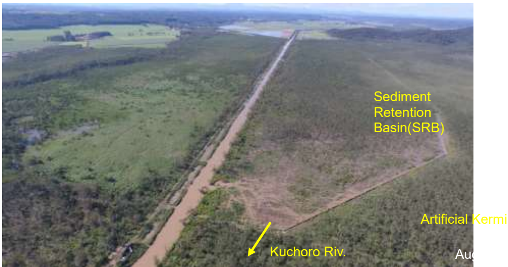
Figure 3. The Sediment Retention Basin (SRB) was constructed on the side of flood plain area at Kuchoro River. A large amount of flood water flowed into the SRB and lots of sediment were deposited there on 2016 flooding.
